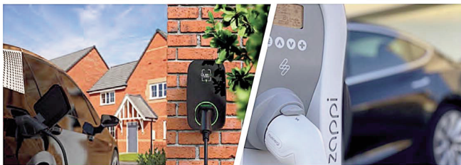
Domestic EV Charging
